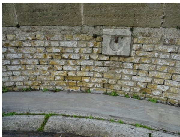
Damaged parapet brickwork
