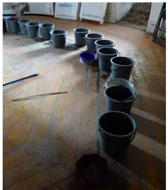
From top: Gun platform showing damaged asphalt; detail of cracked asphalt and failing mortar joint; buckets catching the resulting water ingress.
