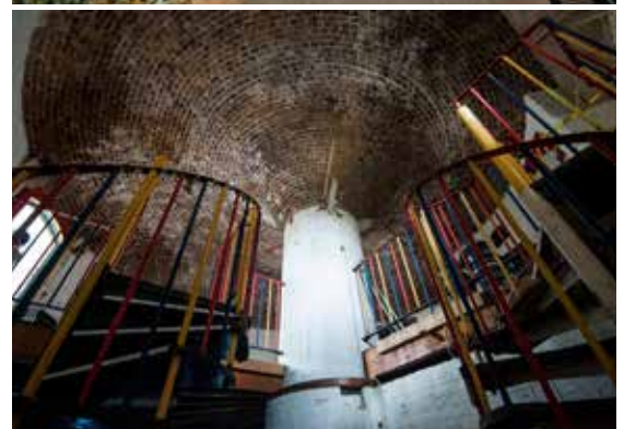
From top: view of The Tower from Wilmington Gardens; visitors enjoying the roof; newspaper article concerning the Wish Tower Café; Wish Tower Café; interior view illustrating construction elements.
