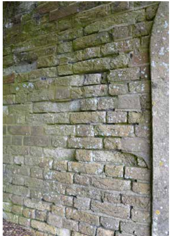
From top: current condition of cementitious render to exterior of the Wish Tower; spalling of bricks in The Moat Wall due to pointing repairs with inappropriate mortar.
