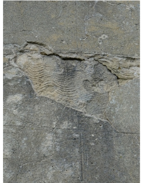
Condition of render from the south-east
