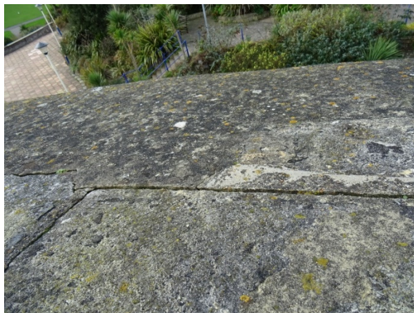
Cracking to parapet render/stone
