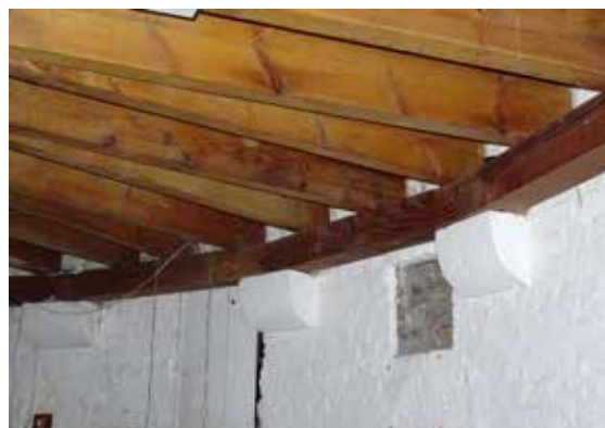
From top: enlarged powder room window in basement; revealed Moat Wall construction on the seaward side; Moat Wall showing courses of brick and greensand on the seaward side; suspended floor structure
