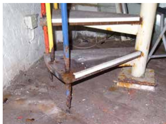
From top: extensive greenery infiltrating Moat Wall; ventilation shaft suspected to be blocked; rotten door surround in magazine/powder room; damp damage to spiral staircase (disused).
