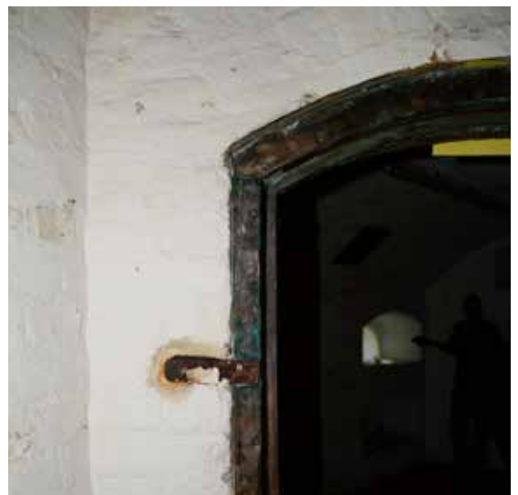
From top: Tower 25 in Dymchurch (not open to the public); interior arched roof (unmodified); copper cladding to the frame of the doorway of the magazine/powder room (unmodified)
