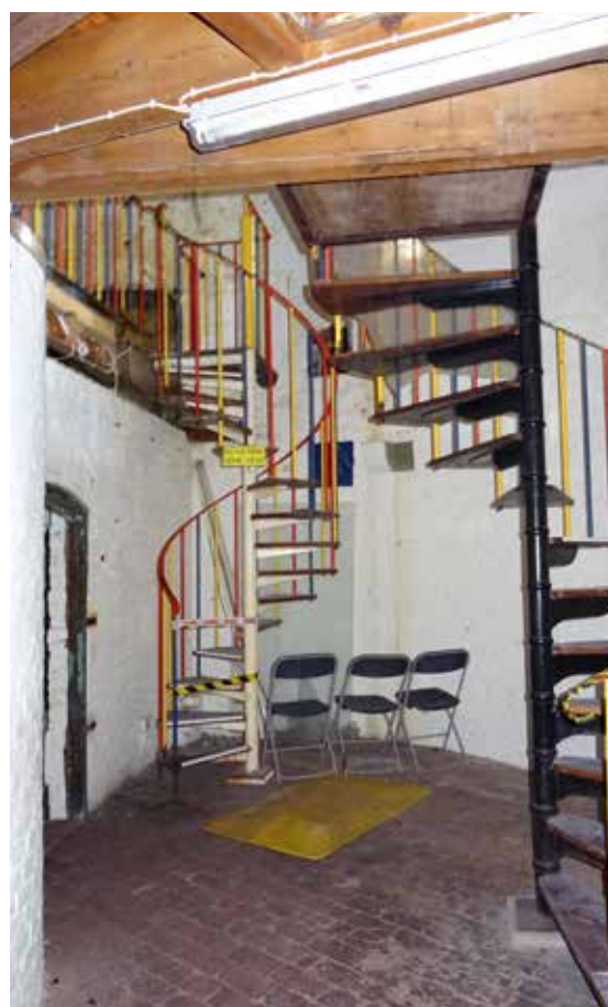
From top: magazine/powder room floor showing original joist position; hatchway to roof which requires additional weatherproofing; brightly painted spiral staircases and C20th electrical intrusions.
