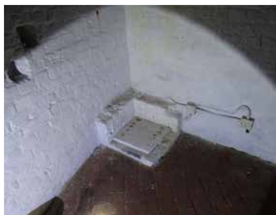
From top: Section through Moat Wall where it was removed which illustrates construction; steel insertion in basement to support spiral staircase; sump of unknown purpose in basement, and intrusion of C20 electrical wiring.
