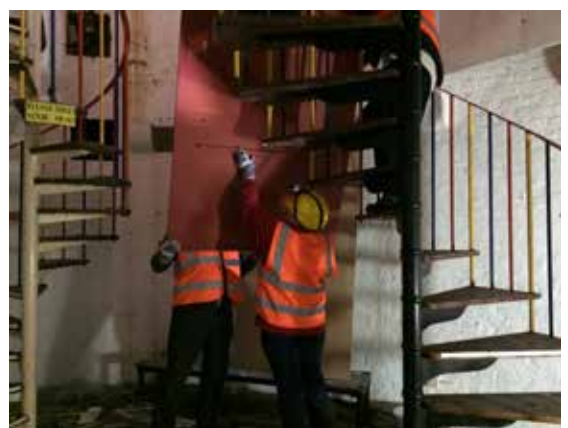
From top: accommodation floor interior showing puppet museum partition before clearance; sheet material being removed outside and inside.
