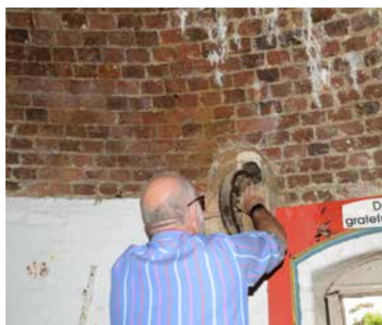
From top: Tours are probably the best form of interpretation but signage is helpful when The Tower is closed; front door showing many alterations; assessing the condition of the drawbridge pulley.
