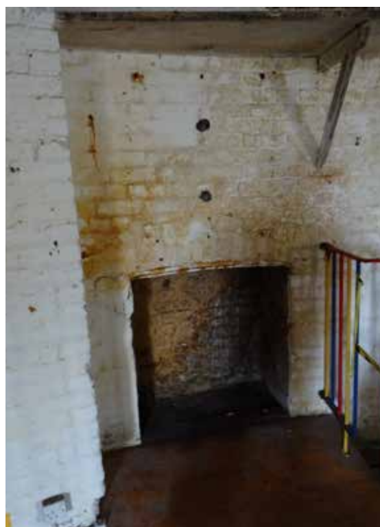
From top: Cracks to the coping of the parapet wall; brick damage and greenery infiltrating brickwork; stalactites from water ingress; damp to fireplace.
