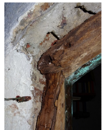
Decayed condition of Magazine door frame
