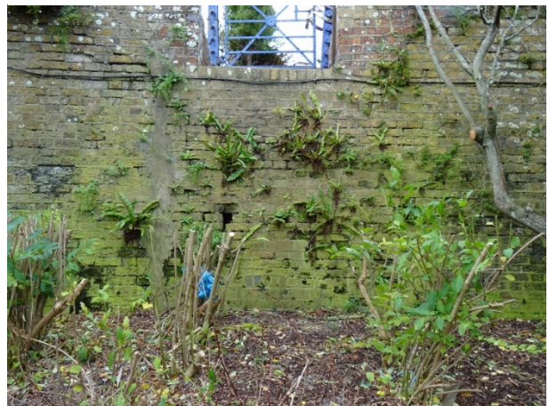
South (internal) face of northern glacis wall showing brickwork erosion
