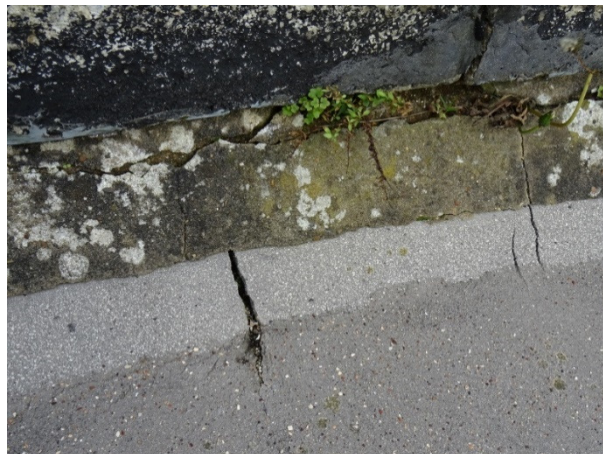
Typical splitting to asphalt
