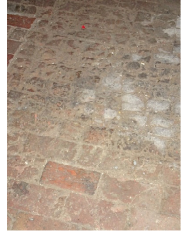
Damaged area of brick floor,
