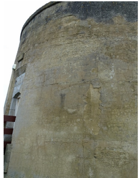
Condition of render from the north-west
