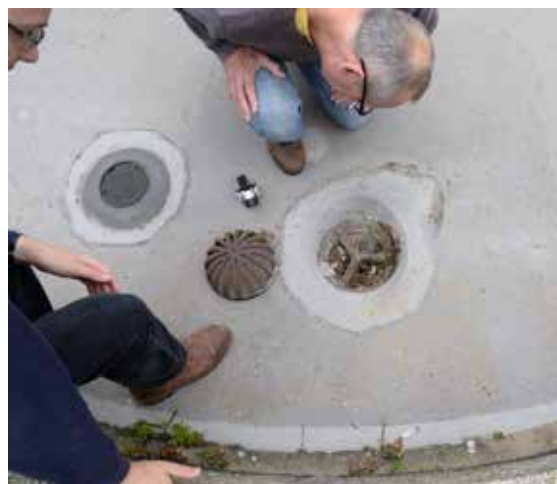
From top: access hatchway to gun platform; gun platform showing damaged asphalt; gun rail with drainage channel; examining roof vents.
