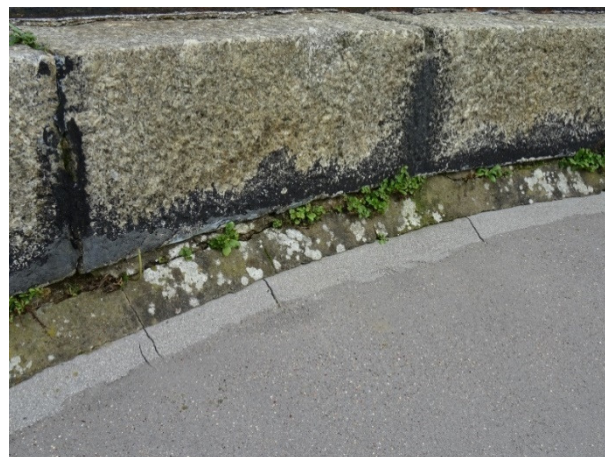
Poor upstand skirt and cement fillet to asphalt
