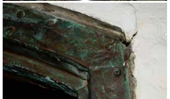
From top: detail of delaminating cementitious render; plant ingrowth to The Moat Wall; garish paint finishes; original copper clad door frame
