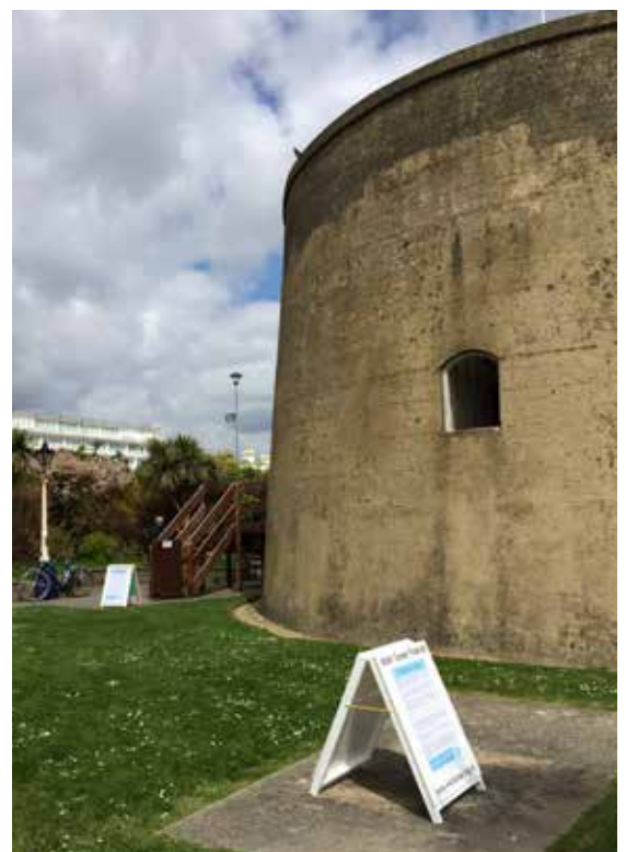
From top: water damage to brick roof arch and C20 intrusion from puppet museum; tower as visitor attraction with rudimentary temporary signage.
