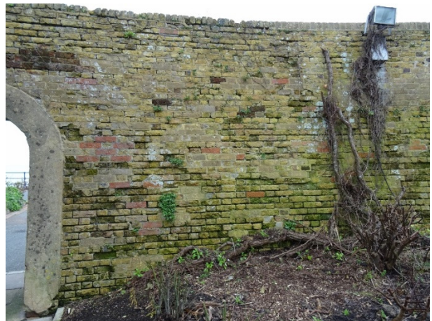
North (internal) face of southern glacis wall showing brickwork erosion
