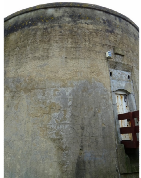
Condition of render from the north-east
